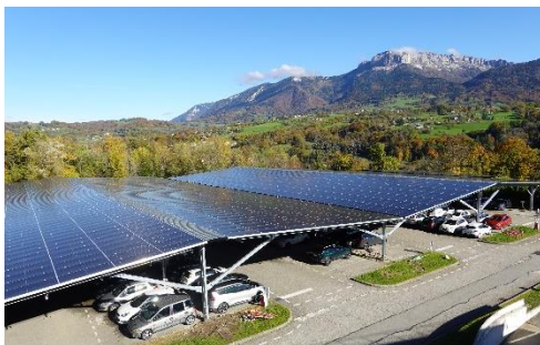
Argonay – photovoltaic panels
