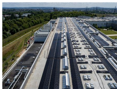
Cergy – photovoltaic panels
